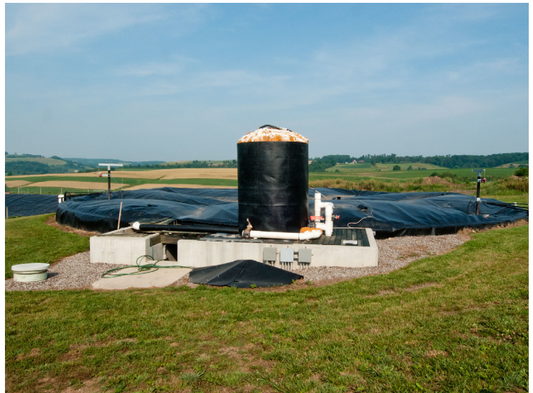
Anaerobic digester on a dairy in Pennsylvania.
