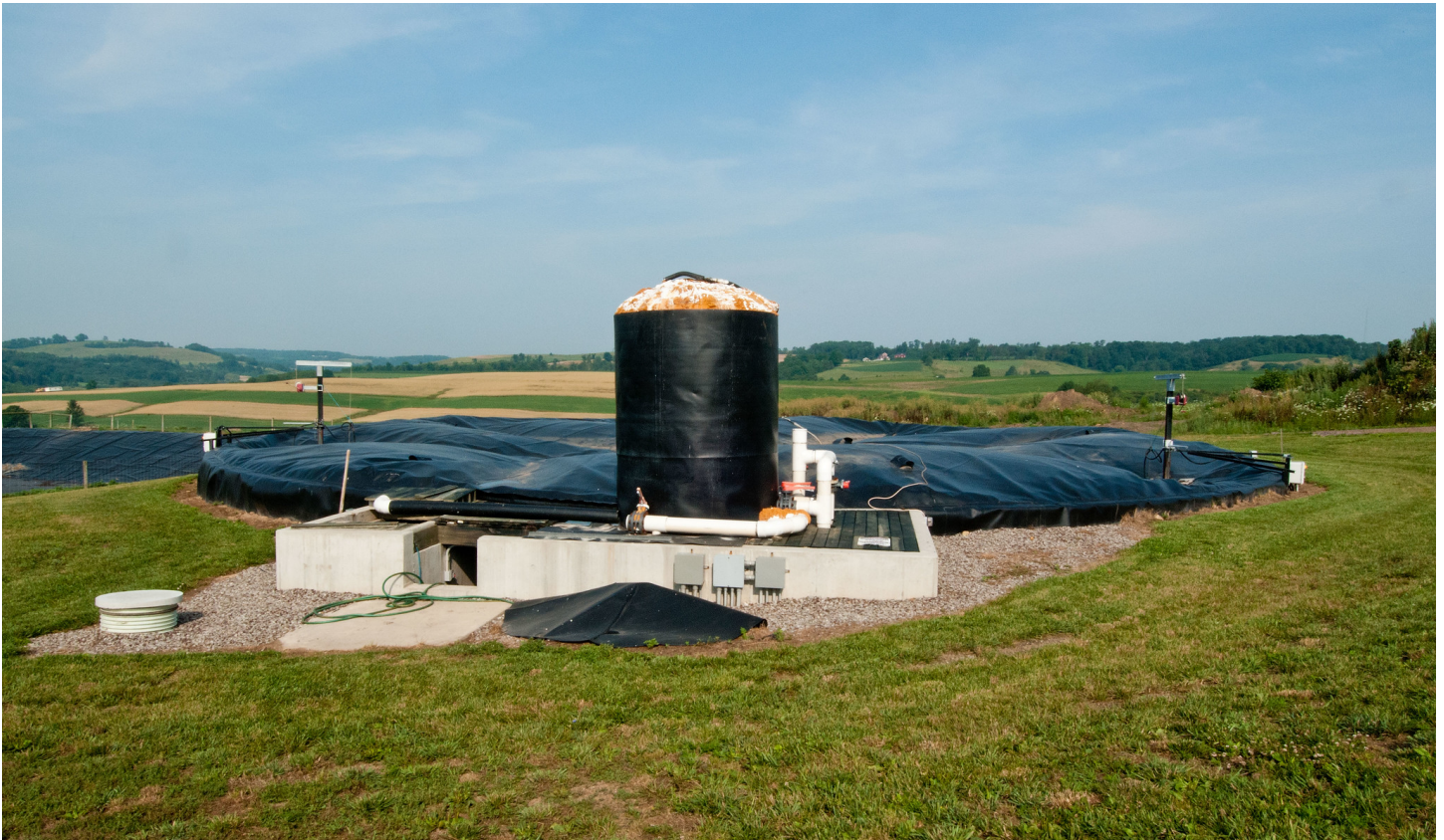
Exterior shot of an anaerobic digester, USDA .
