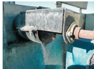
Ash in commercial boilers is automatically removed. It can be reapplied to the soil as a soil amendment.
