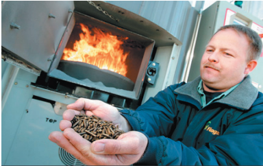
In 2004, Agrecol converted their heating system from LP, and now heats their entire production facilities with native grass pellets
