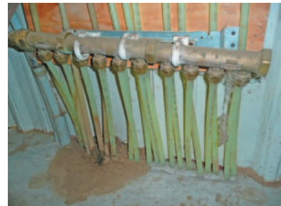
Radiant floor heat system
