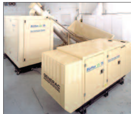
Wood gasification system for small-scale power production.
